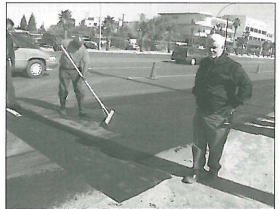
Rubberized Emulsion Aggregate Slurry (REAS) was applied to miles of hurricane-ravaged pavement in Juarez, Mexico.
